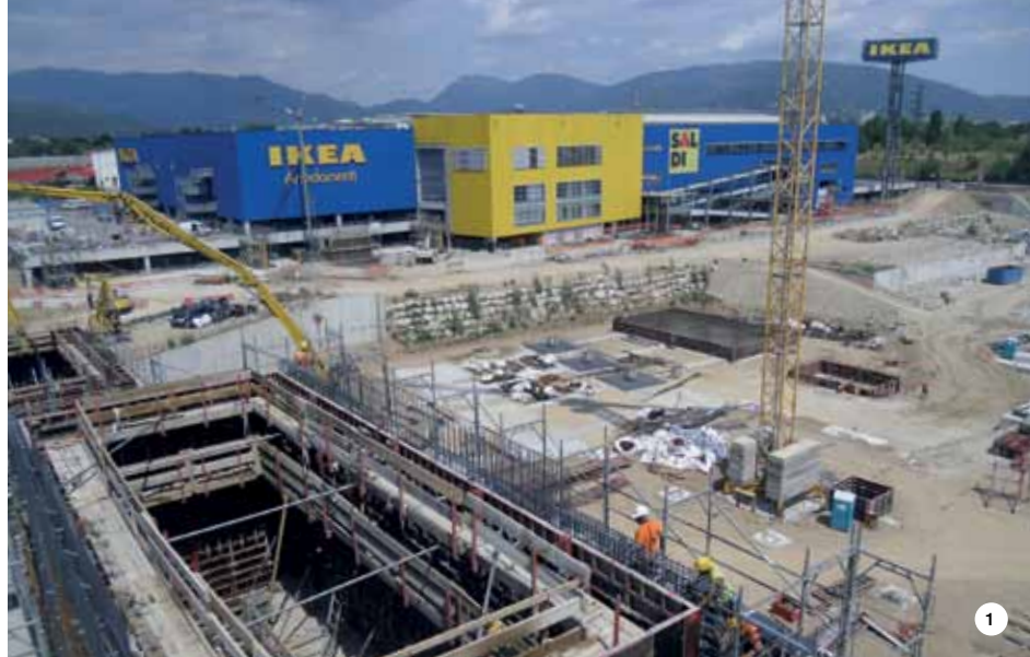
PHOTO 1. Mapei supplied the admixtures EXPANCRETE, MAPECURE SRA 25, DYNAMON XTEND W100 R and DYNAMON XTEND W300 N for the concrete used for the foundation plinths, the walls in the stair and lift wells and the floor slabs.
