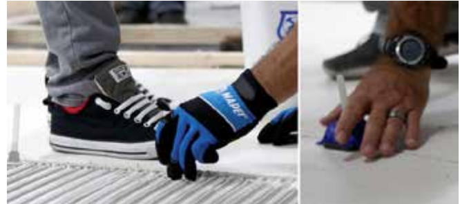
Example of gauged tile over existing tile during a renovation using a mechanical edge-leveling system
