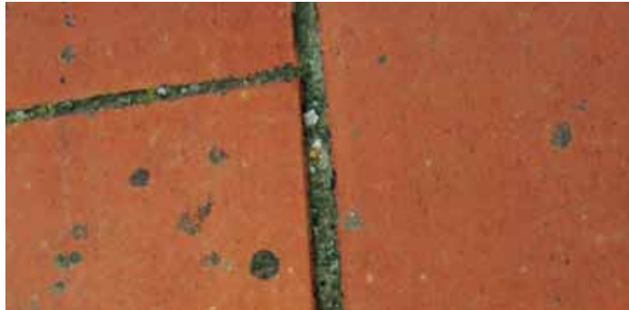
An example of old terracotta floor requiring treatment before applying Aquaflex Roof
