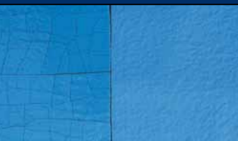
2. Detailed view of cracking of non-flexible paint 2. Elastocolor Waterproof
