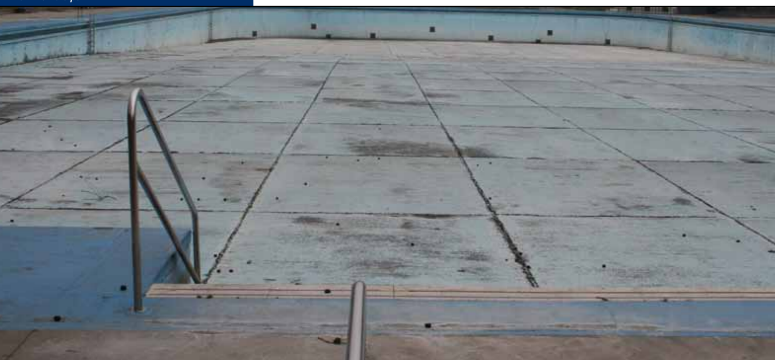
3. Deteriorated swimming pool
