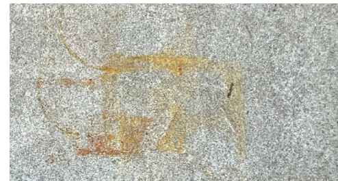
RUST STAIN BEFORE TREATMENT
