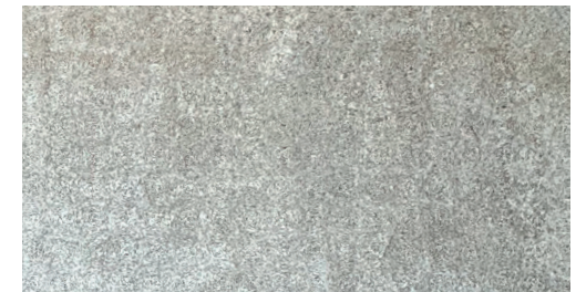
RUST STAIN AFTER TREATMENT
