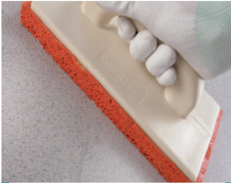
Finishing off the surface of the smoothing and levelling layer with a sponge float
