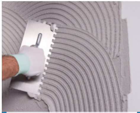
Laying of the first coating of smoothing compound with Mapetherm AR1 GG
