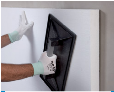
Pressing the panel in place to guarantee a good bond to the substrate
