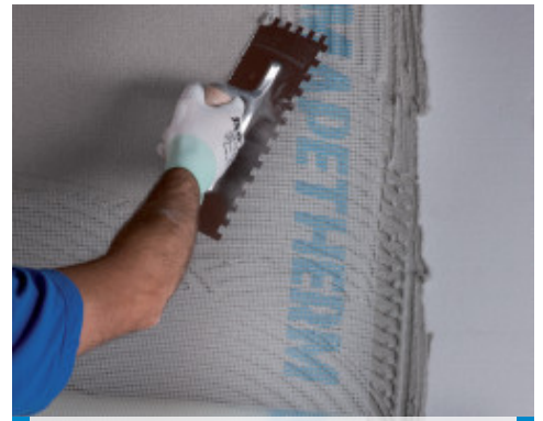
Application of a reinforced smoothing and levelling layer by embedding Mapetherm Net
