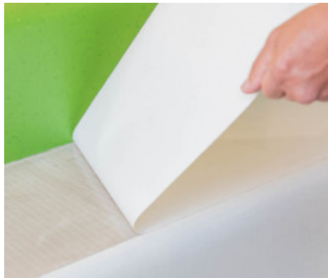
2. Removal of the protective layer from the tread and then from the riser
