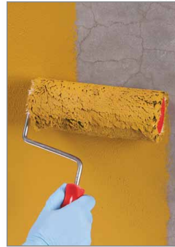
An example of Quarzolite Base Coat applied on a substrate with micro-cracking
