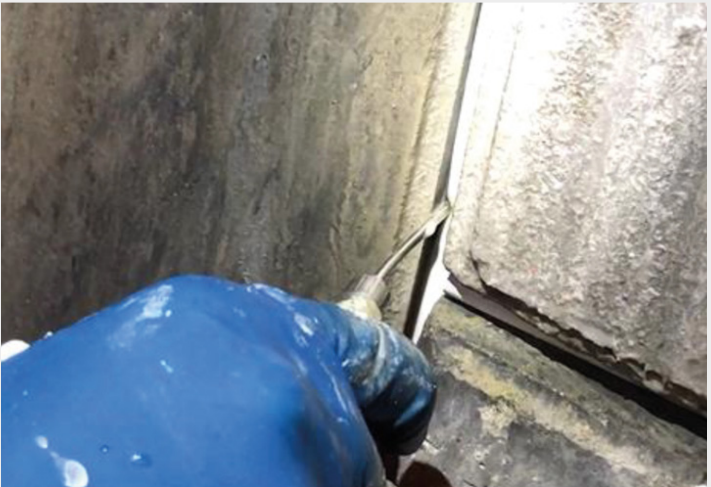
Injection of the cavity between the gasket and MAPEPLAN JOINT by using RESFOAM 1KM HS
