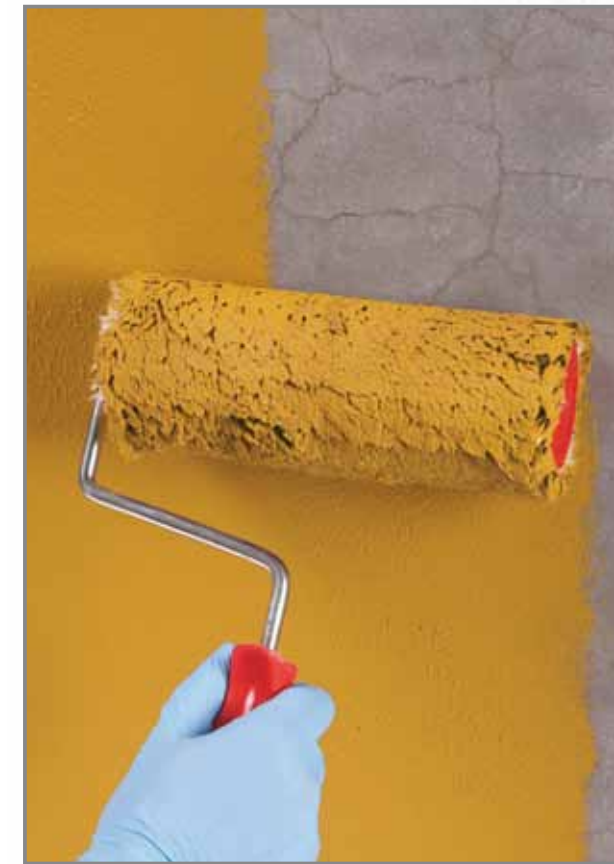
An example of Quarzolite Base Coat applied on a substrate with micro-cracking
