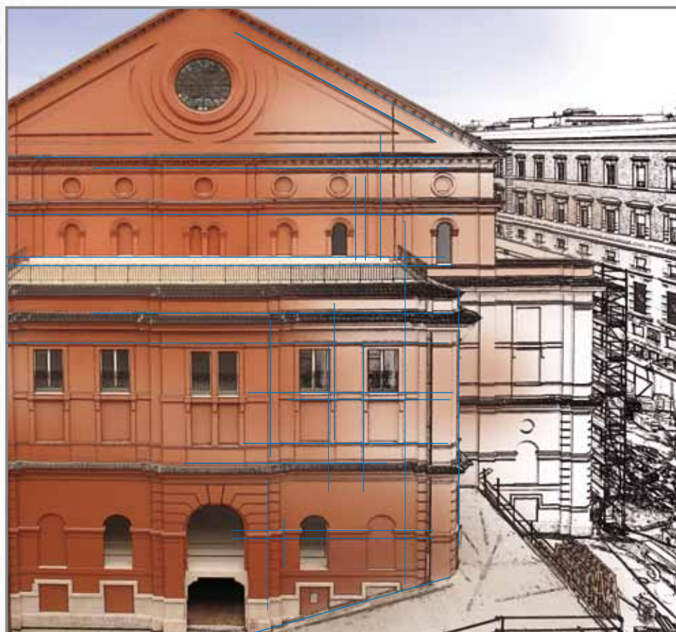
Repair work on the façade of the Petruzzelli Theatre (Bari, Italy) using: Silexcolor Base Coat and Silexcolor Paint
