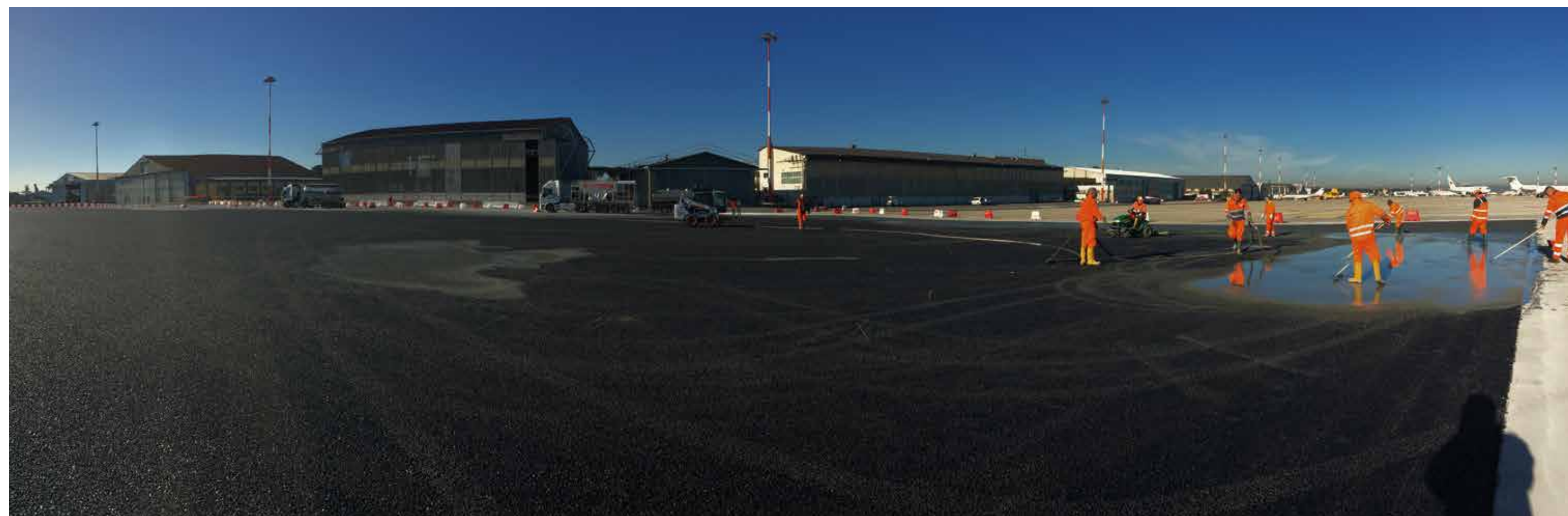
Rome International Airport “Ciampino G. B. Pastine” - Rome - Italy Requalification of the parking area
