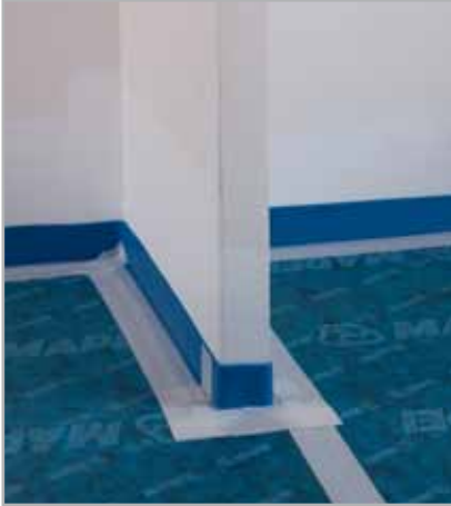
Fig. 4.9 - Floor slab isolated acoustically by laying MAPESENT ROLL, MAPESENT BAND R and MAPESENT TAPE.
