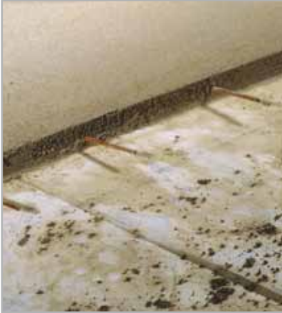
Fig. 7.2 - A screed cut perpendicularly at the point where laying has been interrupted
