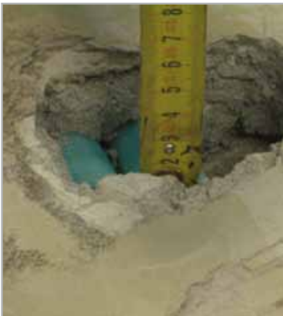
Fig. 8.6 - The thickness of the screed over pipe-work is insufficient (< 30 mm)
