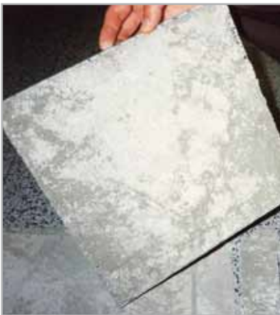
Fig. 3.4 - Ceramic tile detached from a crumbly screed
