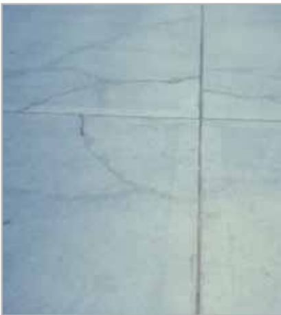
Fig. 3.3 - Serious damage caused by "curling" at an advanced state
