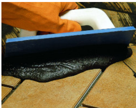
Grouting an external klinker tile floor with Keracolor GG mixed with Fugolastic
