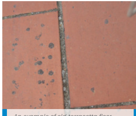
An example of old terracotta floor requiring treatment before applying Aquaflex Roof
