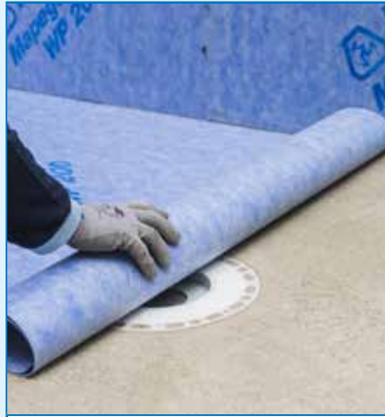
Preliminary positioning of the membrane in order to evaluate the drainage point
