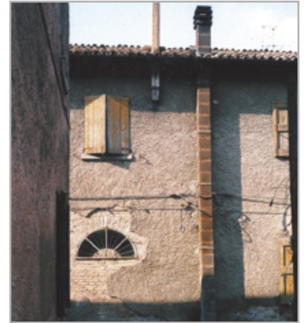
Fig. 6.1 - Masonry building with rising damp
