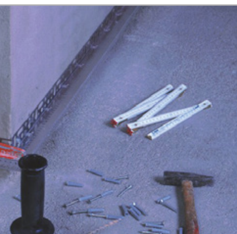
Fig. 6.3 - Positioning the support profiles: make sure they are horizontal using a spirit level
