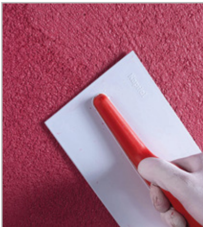
Fig 6.16 - Finishing off the surface of the finishing render with a plastic float
