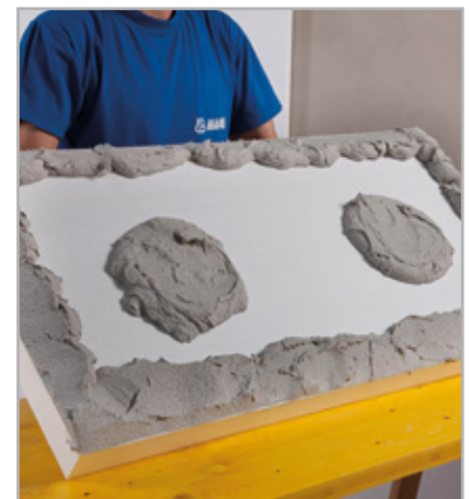
Fig. 6.6 - The back of a panel with beads of adhesive around the edges and spots of adhesive in the middle
