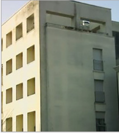
A building without external insulation highlighting thermal bridges in the structure (beams and pillars). Masonry buffer walls damaged by microorganisms due to them being colder
