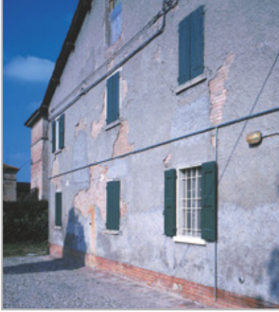
Fig. 6.2 - The areas of detached render must be removed before bonding the insulating panel
