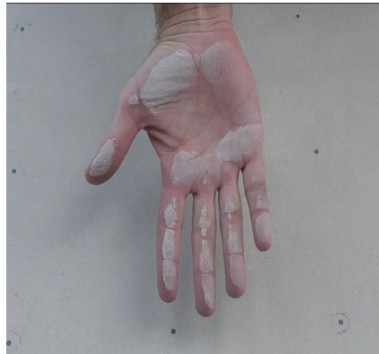
Dusty and weak concrete surface
