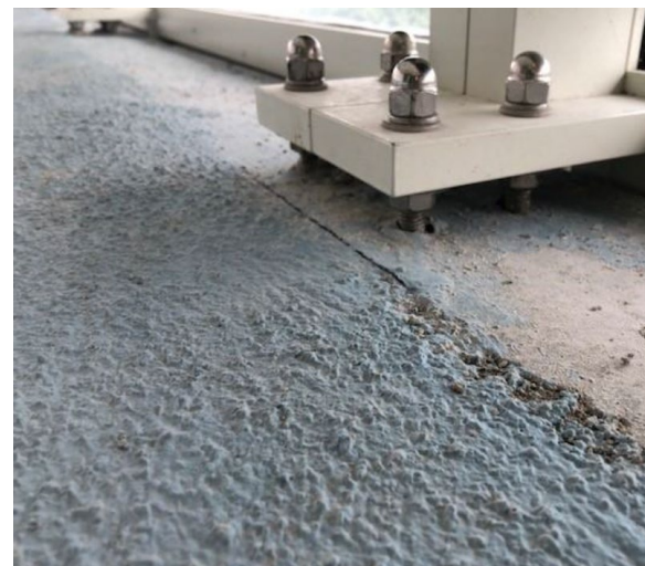
Rough, uneven and contaminated substrate
