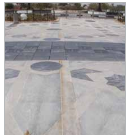
Fig. 4.11 - Example of staining on natural stone installed with acetic cross-linking silicone sealant
