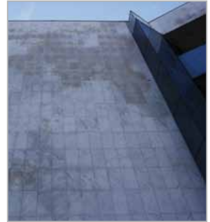
Fig. 2.5 - Example of stains caused by pyrite on white Carrara marble
