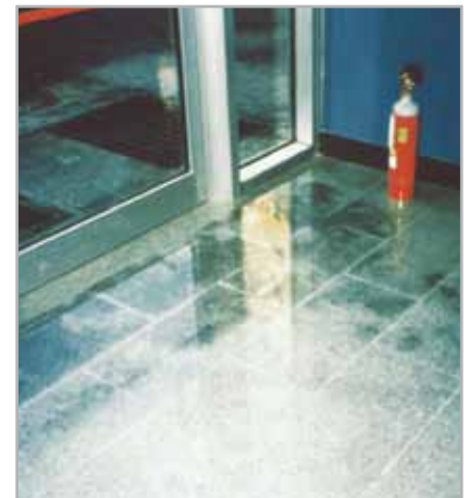
Fig. 2.6 - Example of stains on a granite floor
