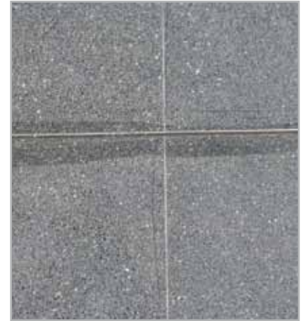
Fig. 4.10 - Example of staining on natural stone installed with acetic cross-linking silicone sealant
