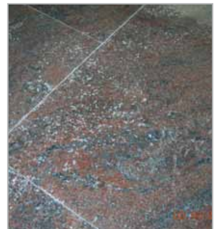
Fig. 2.7 - Example of efflorescence caused by rising damp from the substrate
