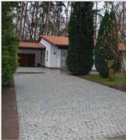
Fig. 5.8 - Example of installation and grouting of porphyry paved floor with MAPEDRAIN MORTAR and MAPEDRAIN 1K GROUT
