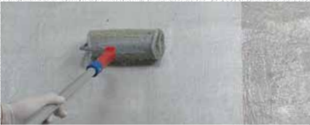
Application of a 2 nd layer of MapeWrap EQ Adhesive to completely impregnate the fabric
