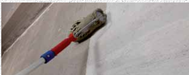
Application of a 1 st layer of MapeWrap EQ Adhesive over existing render
