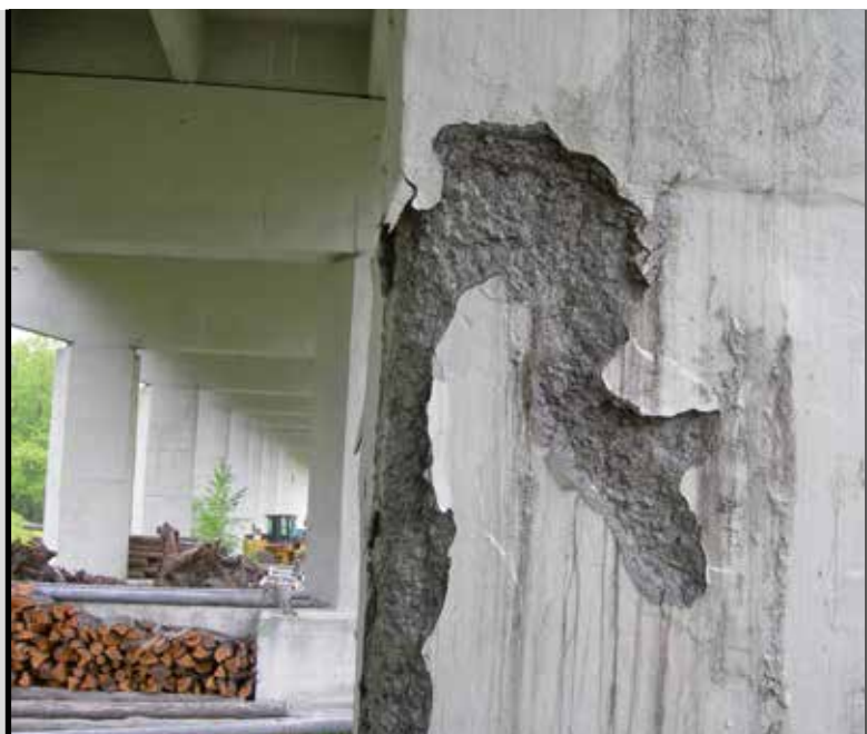
Photo 1 Example of concrete deteriorated by sulphur aggression
