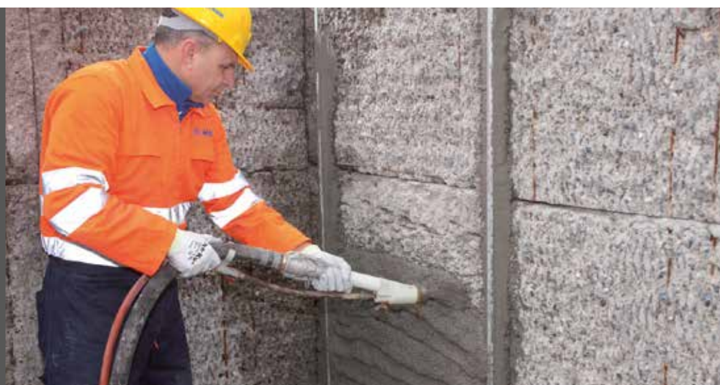
Photo 6 Application by spray of MAPEGROUT 430 , class R3 structural mortar on a concrete structure
