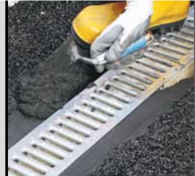
photo 9 Fixing a grated cover on a run-off channel in place using Mapegrout SV T
