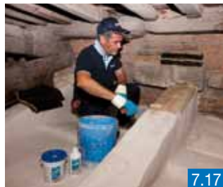
Figures 7.17, 7.18, 7.19, 7.20, 7.21, 7.22, 7.23, 7.24 and 7.25 - Protection applied around reinforcement ribs using fabrics from the MAPEWRAP line
