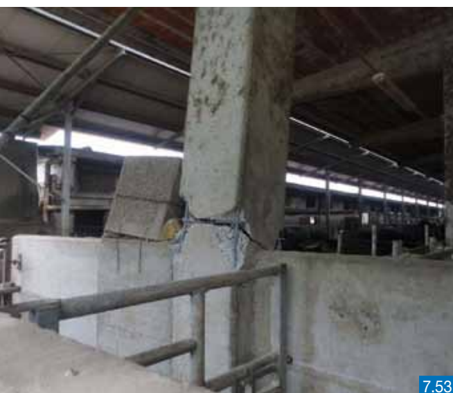
Figures 7.53 and 7.54 - Damage to industrial buildings caused by the earthquake in Emilia (Italy) in 2012
