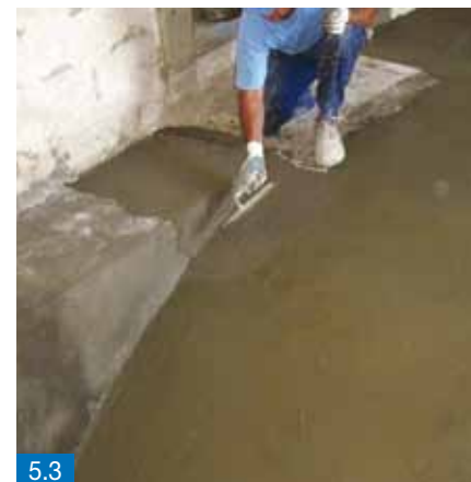
Figures 5.2 and 5.3 - Strengthening on the outer face of stone vaults using PLANITOP HDM MAXI and MAPEGRID G 220
