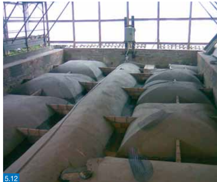
Figures 5.11 and 5.12 - Strengthening system on the outer face of the vaulted roofs of the Church of the Padre Pio Giovane Convent - Serracapriola (Foggia - Italy)
