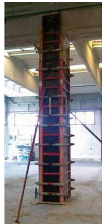
Creating a sleeve around a pillar using PLANITOP HPC + PLANITOP HPC FIBRE
