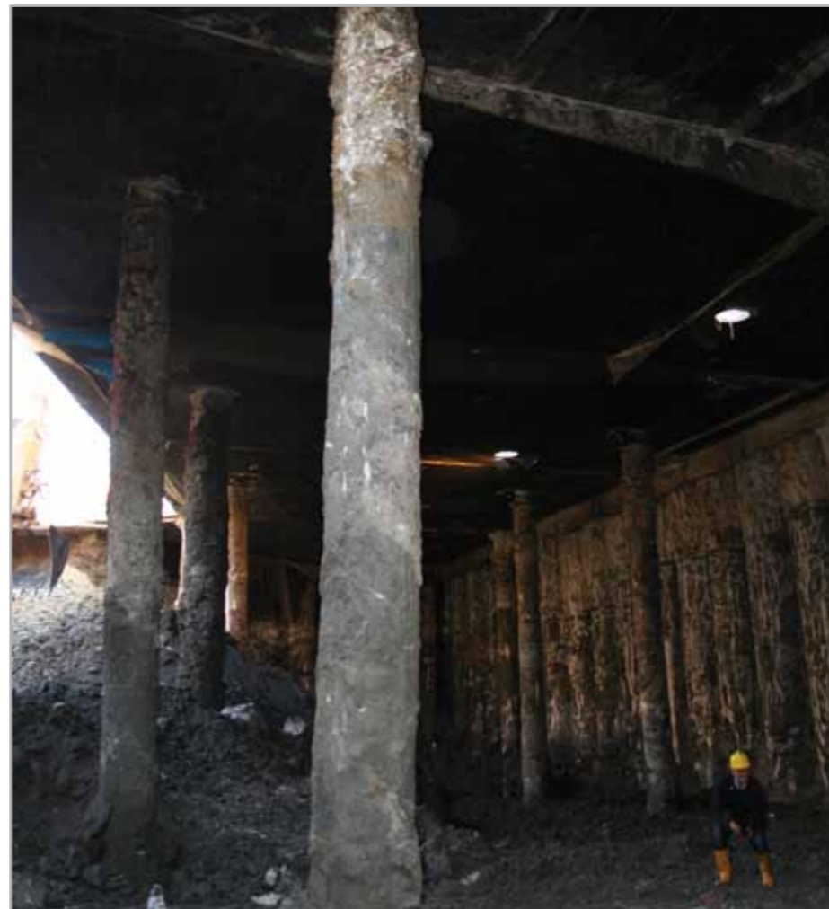
Fig. 4.5 – Example of a Top-Down construction. Excavation work carried out under the reinforced concrete foundation pad cast before excavating
