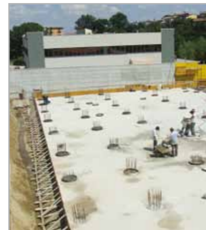
Fig. 7.18 - An overall view of a series of piles during the rebuilding of the heads
