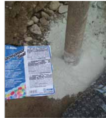
Fig. 7.60a – One of the phases of sealing a pipe which passes through the foundation pad: application of MAPEPROOF SEAL around the pipe
