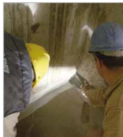
Fig. 8.8c – Application of EPORIP in the fillet joints between horizontal and vertical surfaces and between adjacent walls
