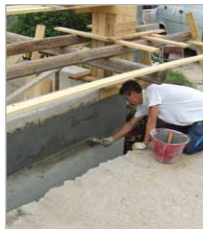
Fig. 7.47 – Application of MAPELASTIC FOUNDATION with a brush on the upper part of a wall before applying MAPEPROOF
