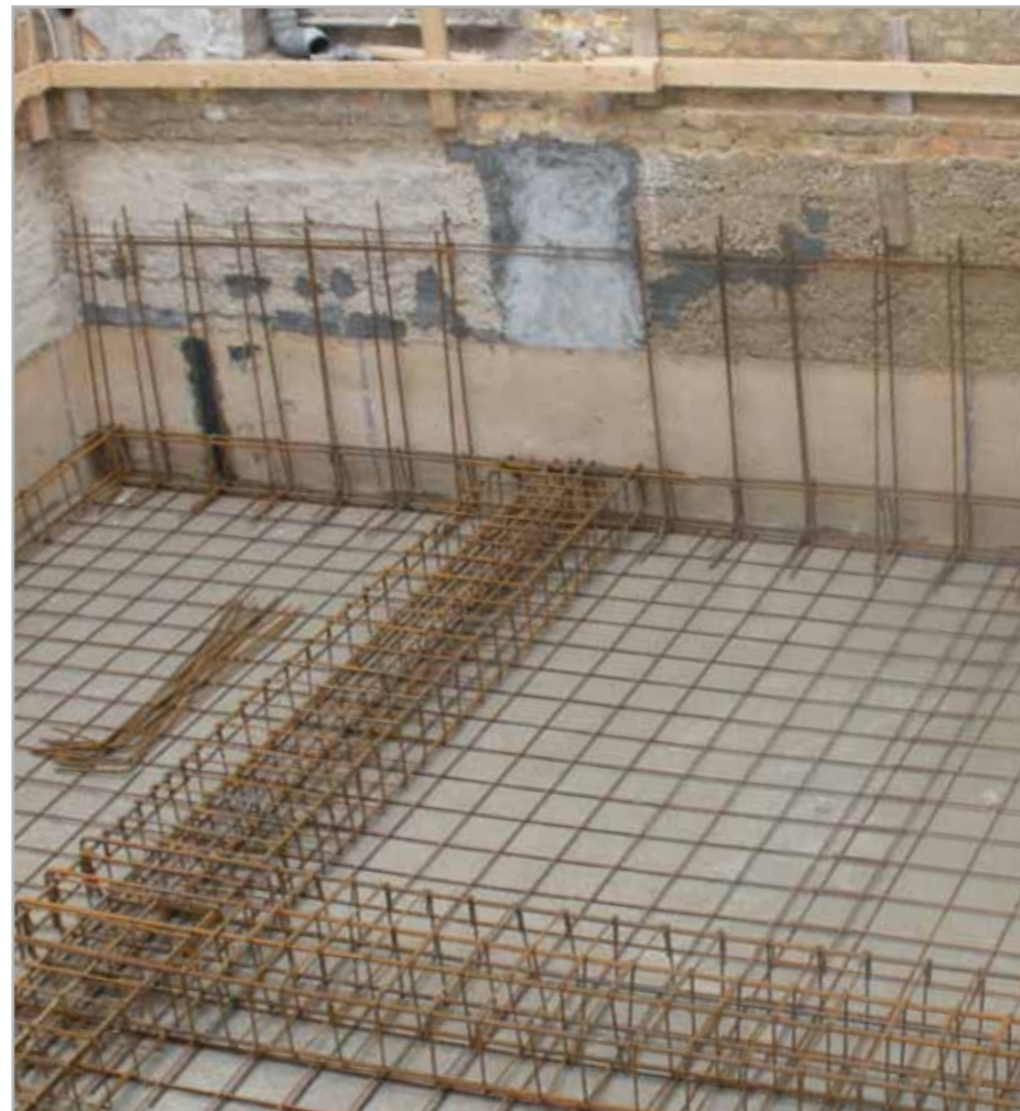
Fig. 8.5b – After laying the sheet on the horizontal surface, the steel reinforcement for casting the reinforced concrete floor slab and counter-wall is placed in position
