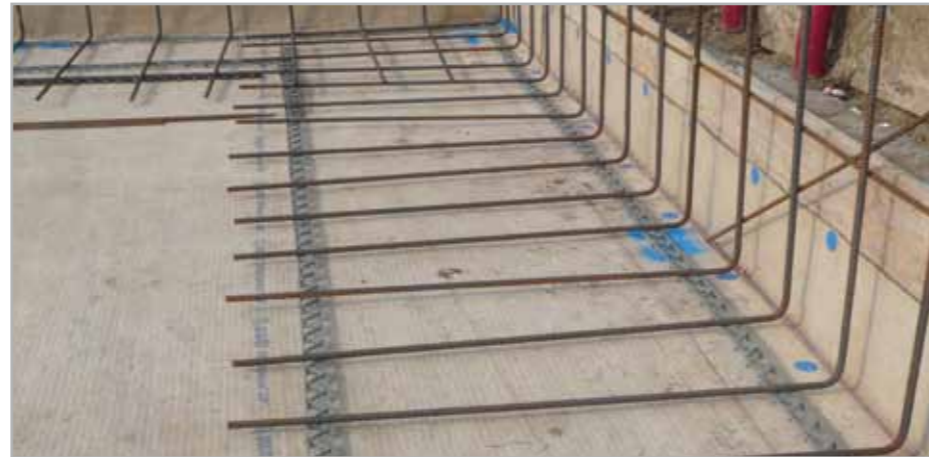
Fig. 7.13 - Metallic reinforcement positioned on MAPEPROOF and separated from the sheets with spacers
