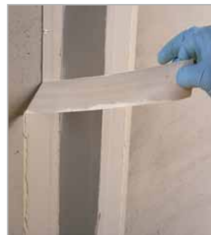
Fig. 7.48e – Before reticulation of ADESILEX PG4, sprinkle quartz sand on the surface and remove the masking tape
