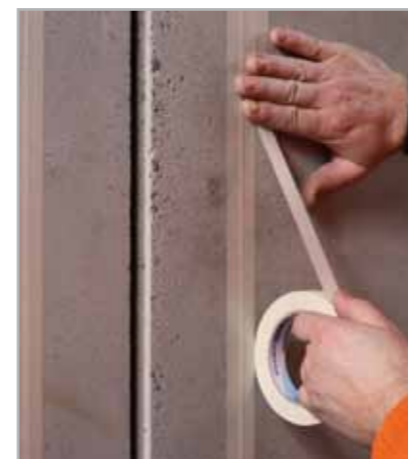
Fig. 7.48a – Phases of waterproofing an expansion joint subject to movements of up to 10 mm with MAPEBAND TPE: to avoid the epoxy adhesive leaving a rough edge, apply masking tape along the sides of the joint
