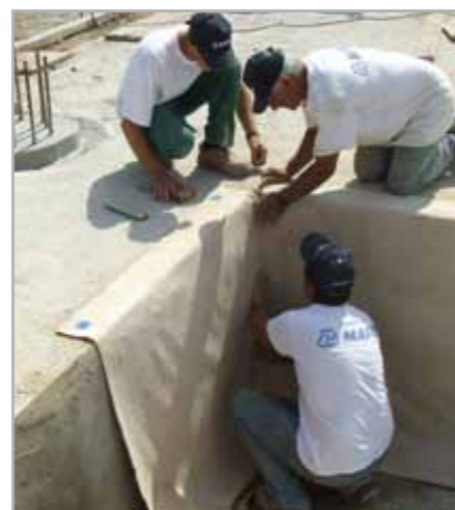
Fig. 7.5a – One of the phases of waterproofing and casting a lift well: application of MAPEPROOF on the side walls of the excavation
