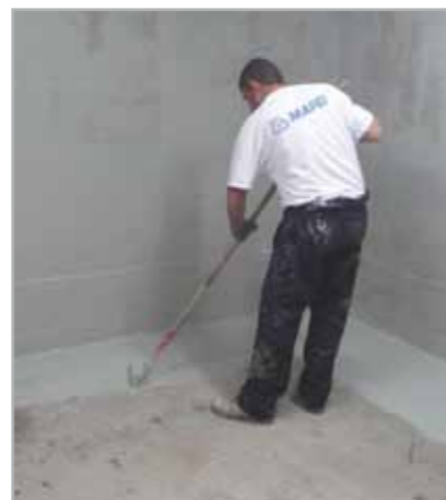
Fig. 8.6a - One of the phases of relining the inside of a room with MAPELASTIC FOUNDATION on the vertical walls and MAPEPROOF on the horizontal surfaces: application of MAPELASTIC FOUNDATION on the vertical walls and on the new lean concrete at a width of at least 50 cm
