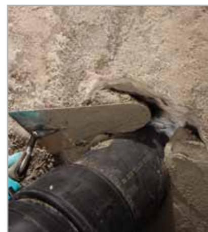
Fig. 8.2 - Sealing a pipe passing through the surface by extruding MAPEPROOF SWELL and then confining the pipe with MAPEGROUT BM
