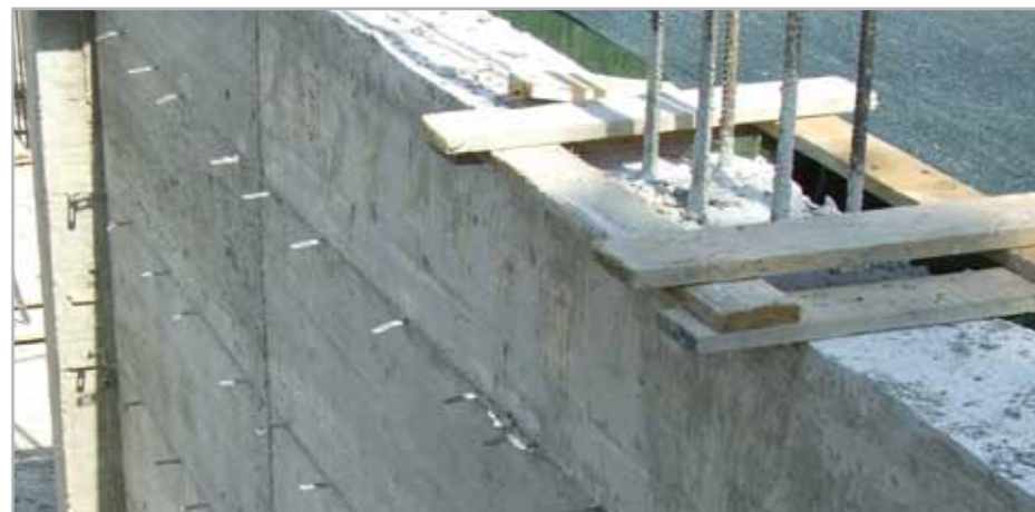
Fig. 7.43 – The blades of the formwork sticking through a reinforced concrete wall before being removed
