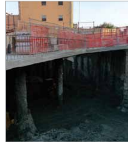
Fig. 7.73 - Excavation work carried out under the reinforced concrete foundation pad cast before excavating
