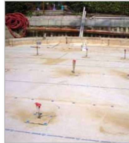
Fig. 7.27 – An overall view of the waterproofing layer on the head of a series of piles
