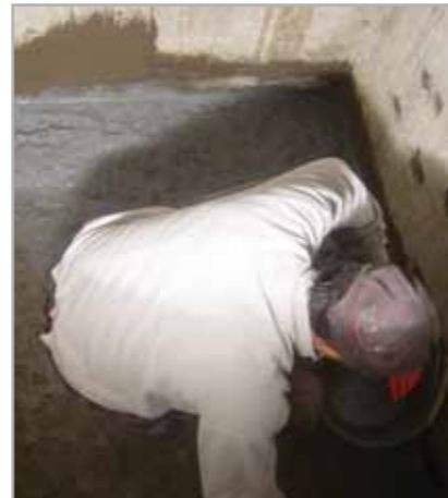
Fig. 8.8a – One of the phases of the installation of waterproof coating with water-repellent IDROSILEX mortar on the horizontal surface and MAPELASTIC FOUNDATION on the vertical and horizontal surfaces: spreading on bonding slurry
