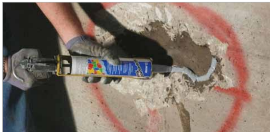
Fig. 8.3 – Extrusion of MAPEPROOF SWELL on a zone damaged by seeping water blocked beforehand with LAMPOSILEX
