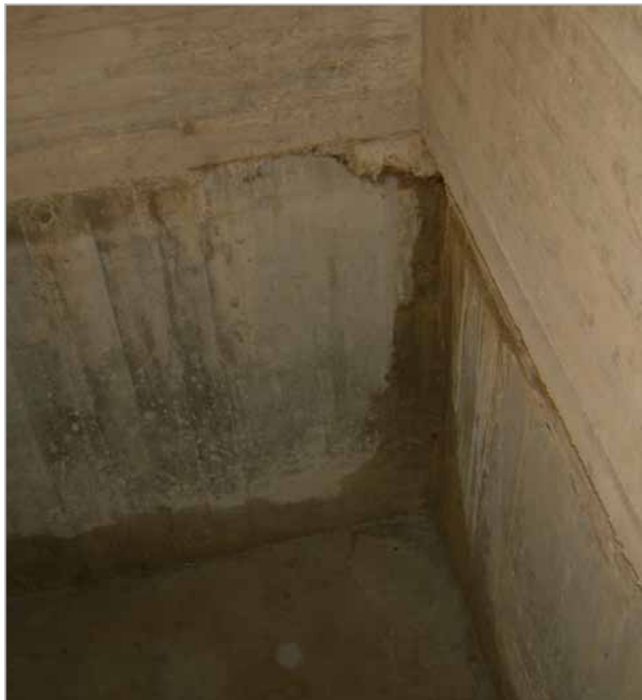
Fig. 8.7 - Infiltrations in correspondence with the construction joints in the reinforced concrete structure for a lift well
