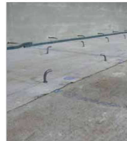
Fig. 8.6d - Metal connectors are required to make the new structure part of the existing one
