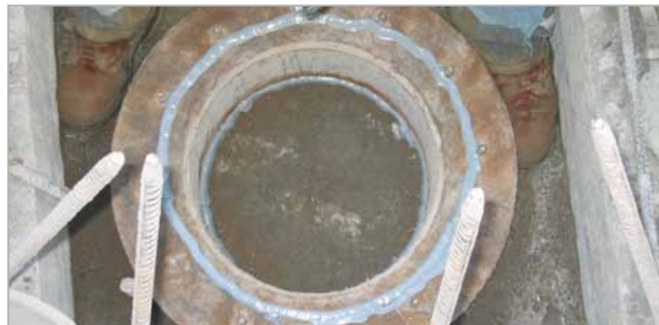
Fig. 7.61 - Extrusion of MAPEPROOF SWELL to seal the joint between a manhole cover and a well
