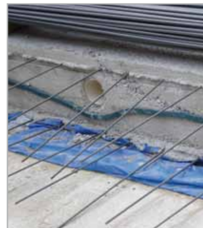
Fig. 7.29 – Sealing a construction joint on a foundation pad with IDROSTOP B25. The protective PE sheet on the strip of MAPEPROOF may be seen protruding from the foundation, which is then overlapped with the adjacent sheet laid before casting the next layer of concrete
