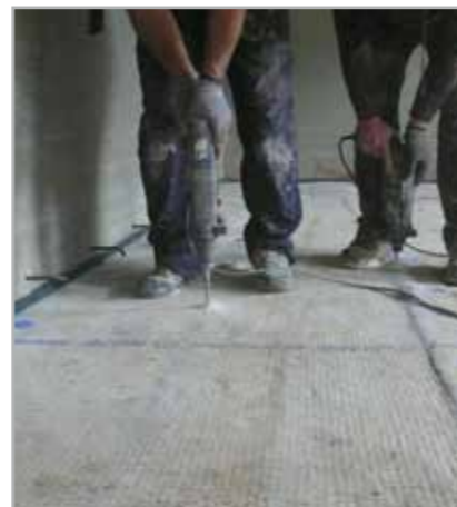
Fig. 8.6c - After laying MAPEPROOF on the lean concrete, make holes to insert the metal connectors
