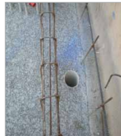
Fig. 7.75 – A hole left in the floor slab to pour concrete into the vertical walls
