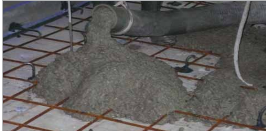
Fig. 8.6h - Casting of the reinforced concrete floor slab, calculated to withstand the hydraulic lift from the groundwater
