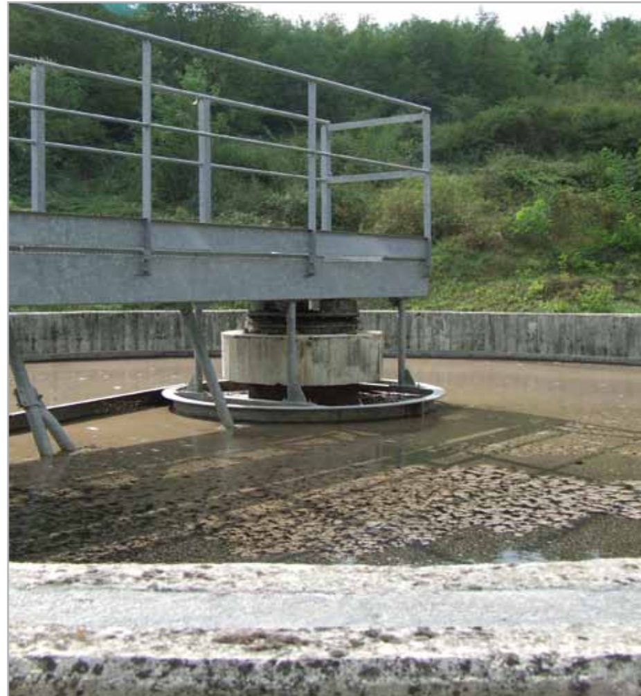
Fig. 7.64 – Sedimentation tank in an advanced state of deterioration
