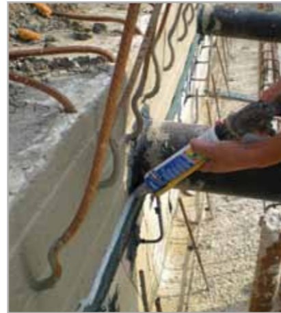
Fig. 7.72 – Extrusion of MAPEPROOF SWELL onto IDROSTOP B25 in the fillet joint between MAPELASTIC FOUNDATION and MAPEPROOF
