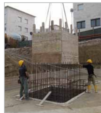
Fig. 7.5e – Positioning wooden formwork before sealing construction joints between a foundation pad and the walls using IDROSTOP B25
