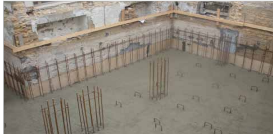
Fig. 8.5c - Reinforced concrete floor slab cast on the MAPEPROOF at a thickness calculated to withstand hydraulic lift from the groundwater
