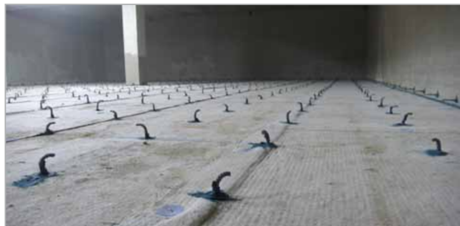
Fig. 8.6g - Metal connectors grouted before positioning the steel reinforcement for the new floor slab to be installed
