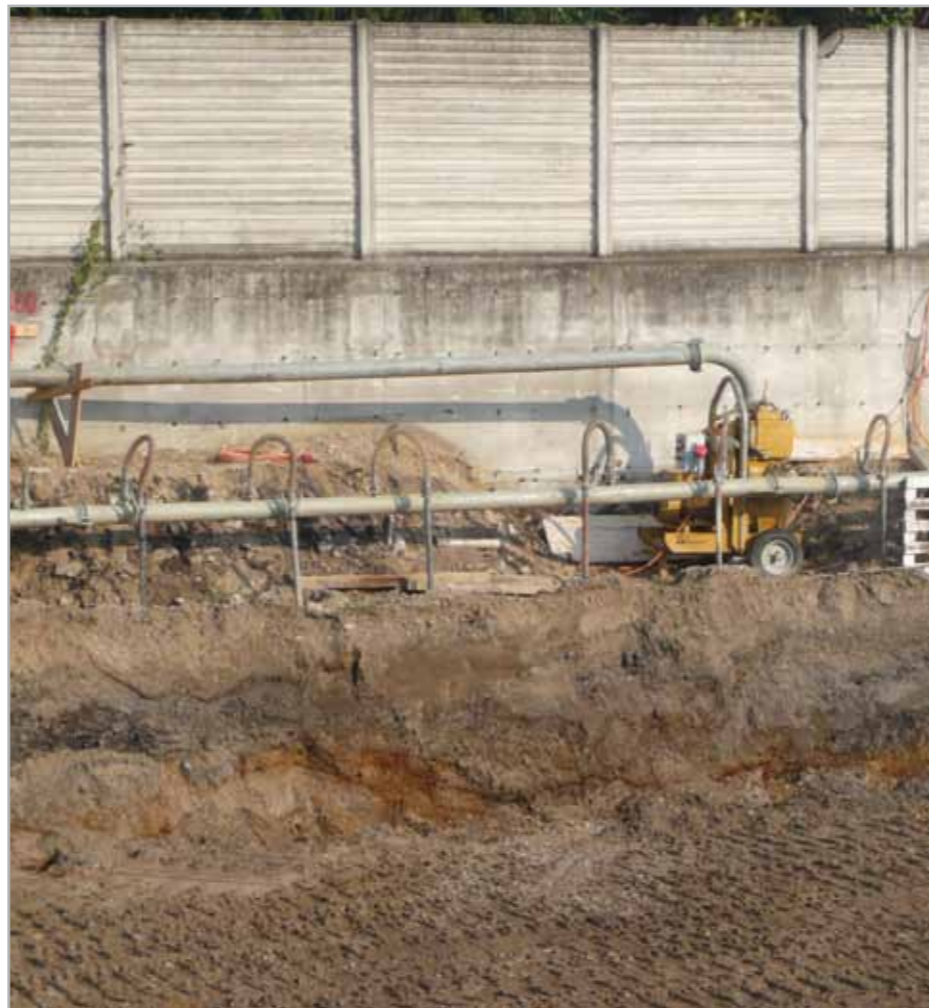
Fig. 3.7 – Centrifugal pump used in a wellpoint system
