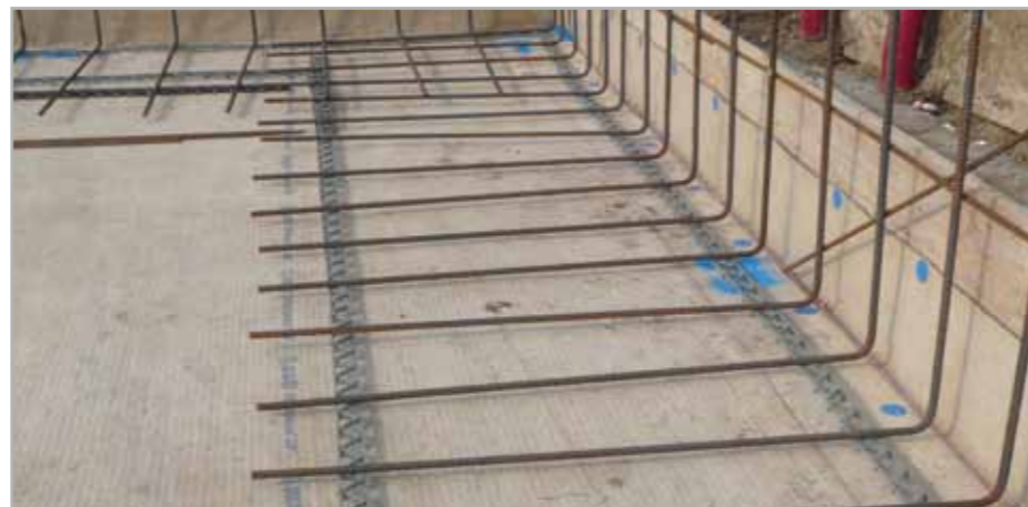
Fig. 7.13 – Metallic reinforcement positioned on MAPEPROOF and separated from the sheets with spacers
