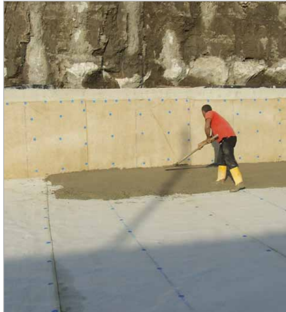
Fig. 7.9 – One of the phases of casting the protective layer of concrete on MAPEPROOF, using concrete with the same Rck as that of the foundation pad
