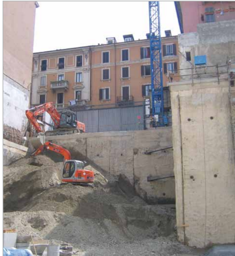
Fig. 1.1 – Phases of an excavation for construction work carried out below ground level in a built-up area
