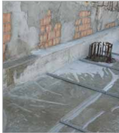
Fig. 7.66 - Application of a sheet of PE to form a floor slab with a regular inner side
