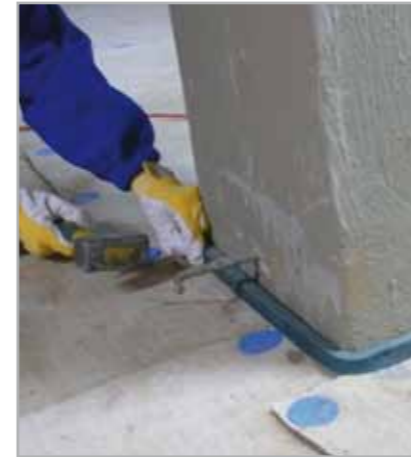
Fig. 8.6e - Lay IDROSTOP B25 in correspondence with the joints between MAPELASTIC FOUNDATION and MAPEPROOF
