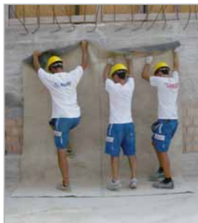
Fig. 7.68 - Bentonite sheet laid on the vertical surface and then hemmed over onto the horizontal surface
