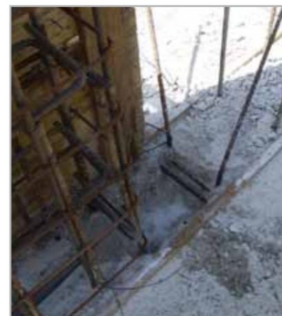
Fig. 7.56b – Demolition to a depth of 15 cm from the upper part of the foundation pad
