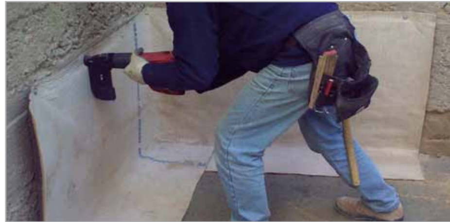
Fig. 8.5a – One of the phases of lining the inside of a room with MAPEPROOF on the horizontal and vertical surfaces: application of MAPEPROOF on the lower part of the vertical walls with the sheet hemmed over onto the lean concrete
