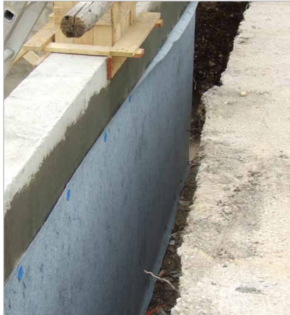
Fig. 7.49 – Protection of the waterproofing material when re-filling by applying 250 g/m 2 non woven fabric in a continuous thread
