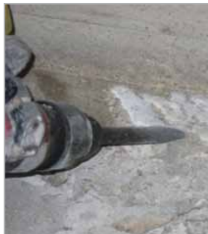
Fig. 8.1a - One of the phases of sealing a construction joint: mechanical demolition around a construction joint to a depth of approximately 6 cm
