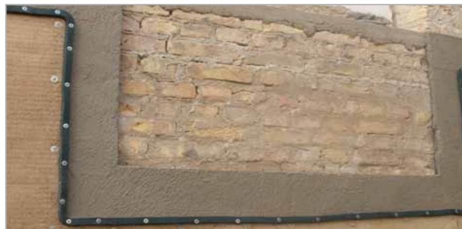
Fig. 8.5d - Sealing a fillet joint between MAPEPROOF and MAPELASTIC FOUNDATION with IDROSTOP B25
