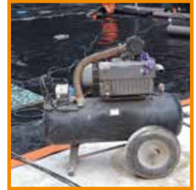
V Vacuum Pump Test
