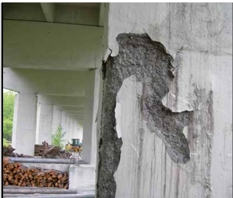
Photo 1 Example of concrete deteriorated by sulphur aggression
