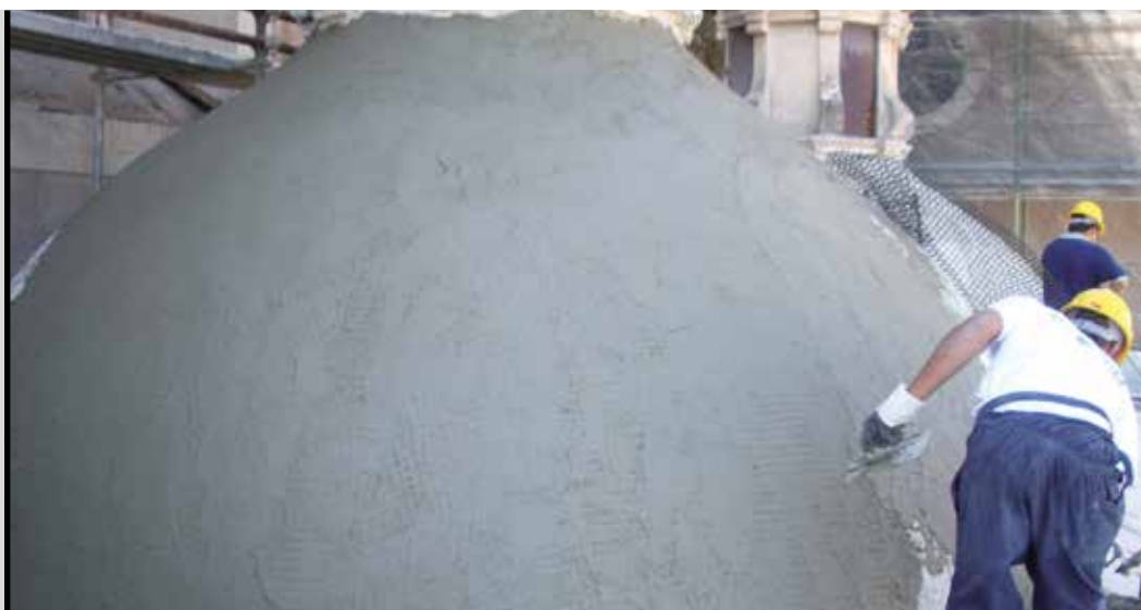
Photo 5 Strengthening of a concrete structure with PLANITOP HDM + MAPEGRID G220 , non-structural class R2 mortar
