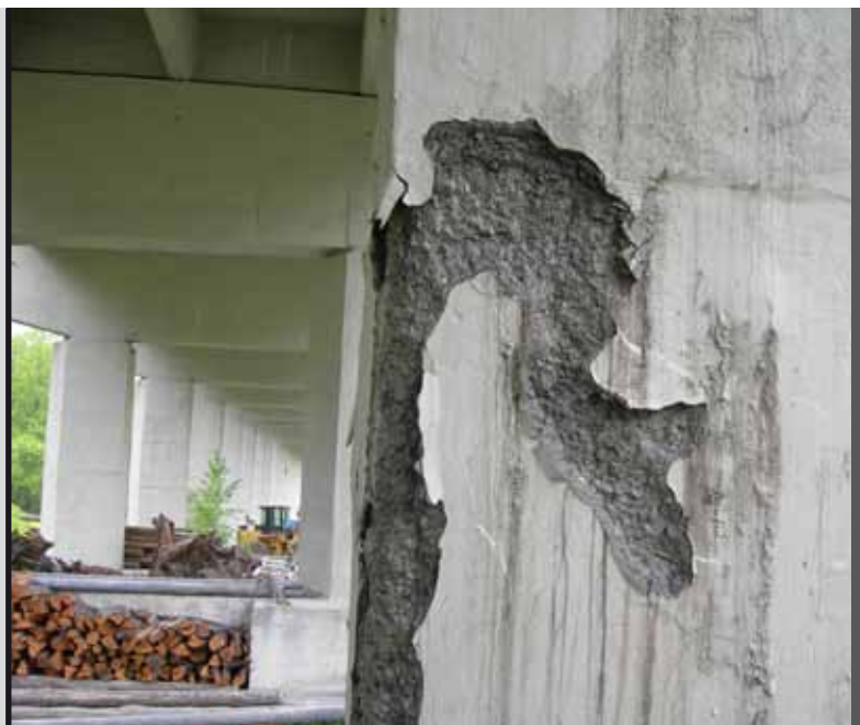
Photo 1 Example of concrete deteriorated by sulphur aggression
