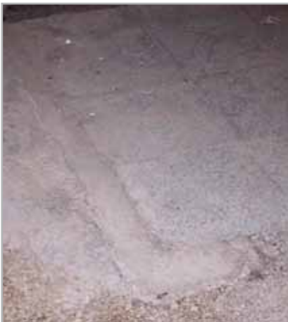
Fig. 7.3 - Sealing a chase in existing flooring by applying bonding slurry on the contact surfaces between the existing and repaired surfaces
