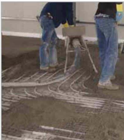
Fig. 4.7 - Laying a screed with embedded heated elements for an underfloor heating system.
