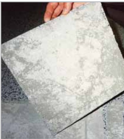
Fig. 3.4 - Ceramic tile detached from a crumbly screed
