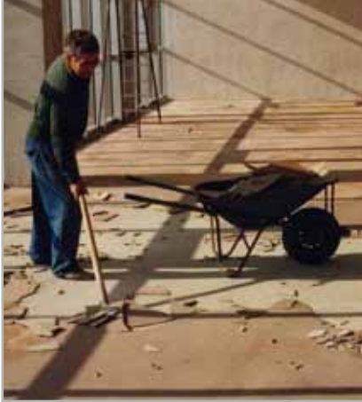
Fig. 8.10 - ULTRAPLAN detached from a screed with surface bleeding
