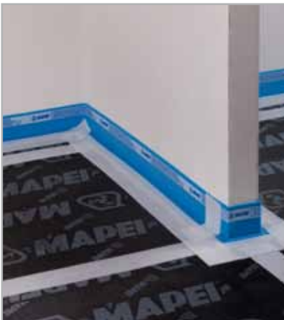
Fig. 4.10 - Floor slab isolated acoustically by laying MAPESENT PANEL, MAPESENT BAND R and MAPESENT TAPE.
