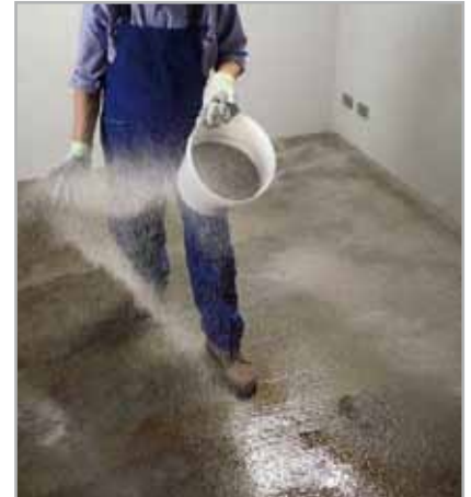
Fig. 8.12 - Dusting the surface of a screed with sand after applying a coat of PRIMER MF
