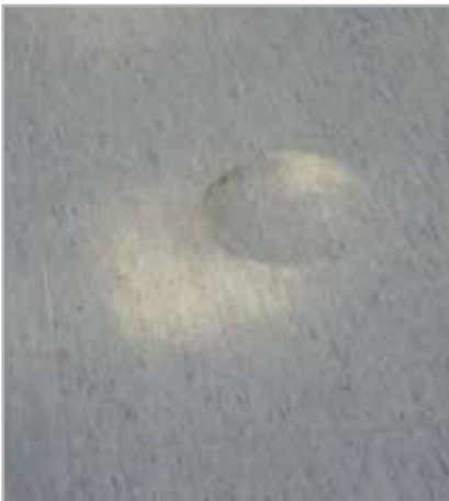
Fig. 8.5 - A depression in an underfloor screed in correspondence with pipe-work
