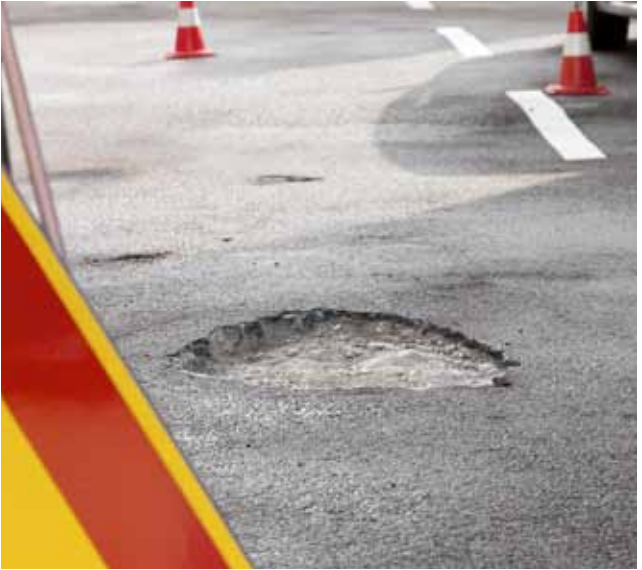
1. Holes in a road ready to be repaired
