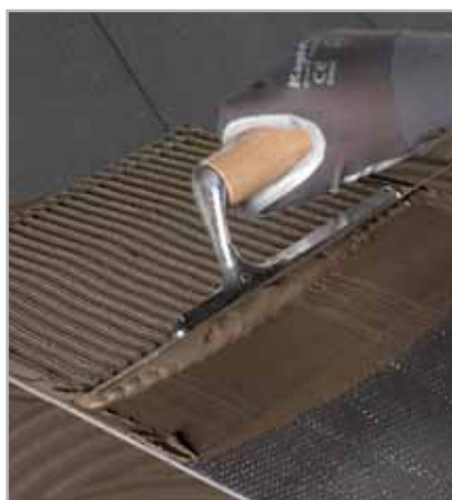
Fig. 7.2 - Laying on floors: spreading the adhesive on the back of the tile
