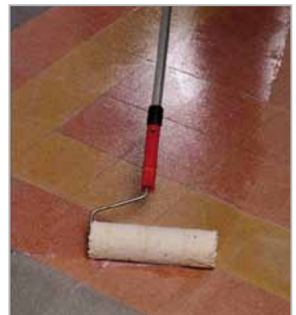
Fig. 5.3 - Application of ECO PRIM T with a roller on an old terrazzo floor before levelling the surface
