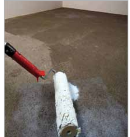
Fig. 5.1 - Application of PRIMER G diluted at a rate of 1:1 with a roller on a cementitious screed before levelling the surface
