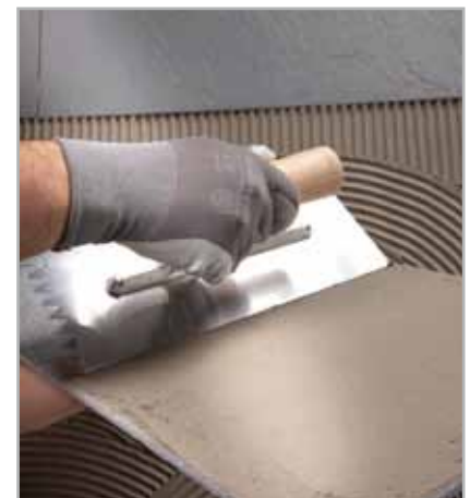
Fig. 7.5 - Fixing to walls: applying the adhesive on the back of a tile
