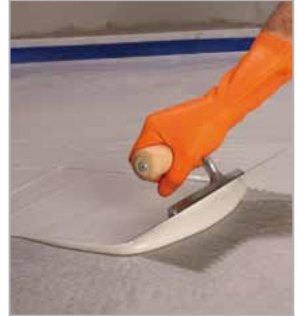
Fig. 7.16 - Application of a second coat of MONOLASTIC by trowel on MAPETEX SEL
