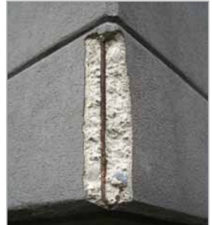
Fig. 6.1 - Corner of the concrete expelled due to corrosion of the reinforcement steel
