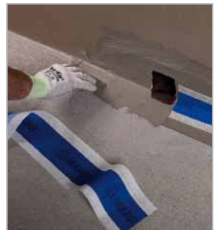
Fig. 5.66 - Application of MAPELASTIC or MAPELASTIC SMART in the wall-floor fillet joint to apply MAPEBAND around DRAIN FRONT
