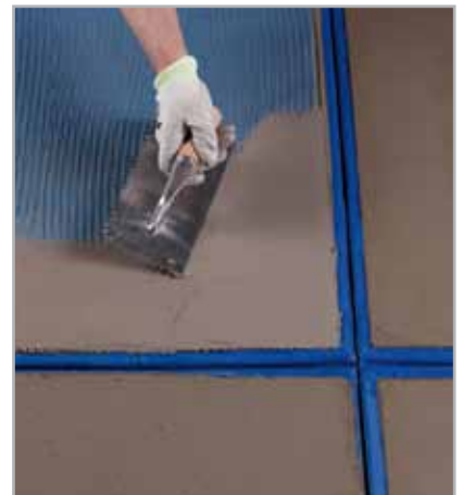
5.71 - Application of MAPENET 150 starting from the control joint followed by embedding MAPENET 150 in the first fresh layer of MAPELASTIC
