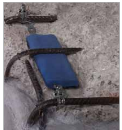
Fig. 6.3 - MAPESHIELD I applied on the reinforcement steel of an element under repair
