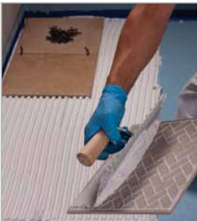
Fig. 8.5 - Spreading the adhesive on the back of a tile to avoid the formation of gaps under the coating
