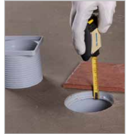
Fig. 8.1 - Measuring the height to position the floor drain flush with the surface of the finished floor
