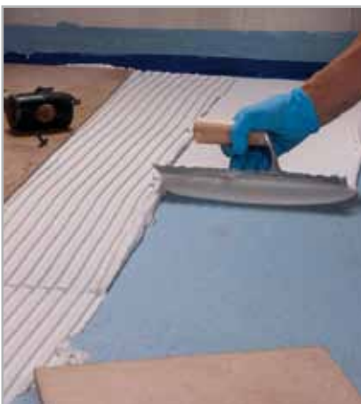
Fig. 8.6 - Bonding the tiles on perfectly dry MAPELASTIC AQUADEFENSE with a class C2 adhesive
