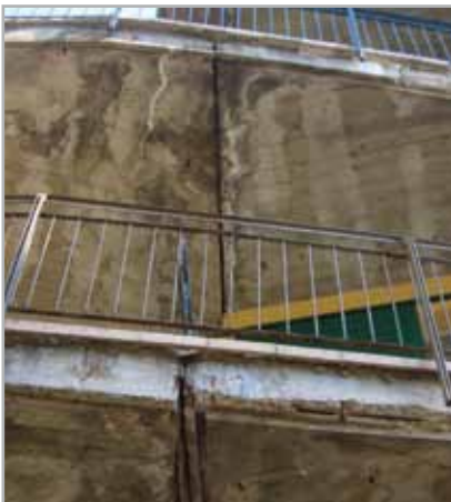
Fig. 5.3 - Deteriorated structural joint
