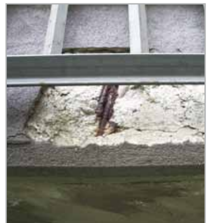
Fig. 6.2 - Deteriorated front edge of a balcony
