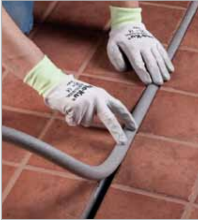
Fig. 9.4 - Inserting MAPEFOAM cord in the structural joint to regulate the thickness of MAPEFLEX PU40
