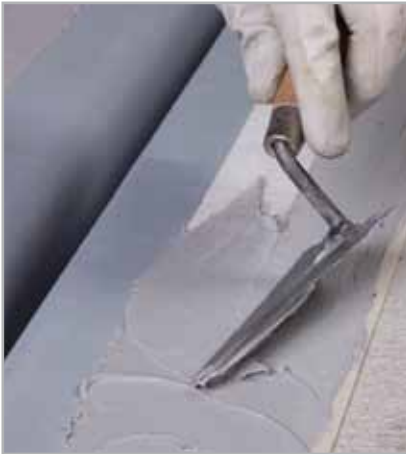
Fig. 5.44 - After laying MAPEBAND TPE on fresh ADESILEX PG4 apply the second layer
