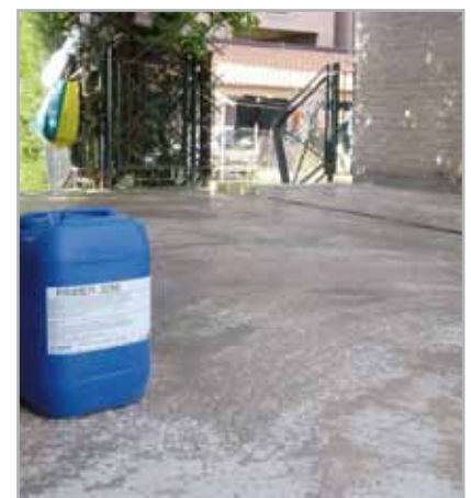
Fig. 5.30 - Applying PRIMER 3296 to consolidate the screed with a sprinkling of sand on the surface
