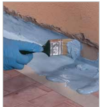
Fig. 5.24 - MAPELASTIC AQUADEFENSE applied by brush on a floor-wall fillet joint before applying MAPEBAND
