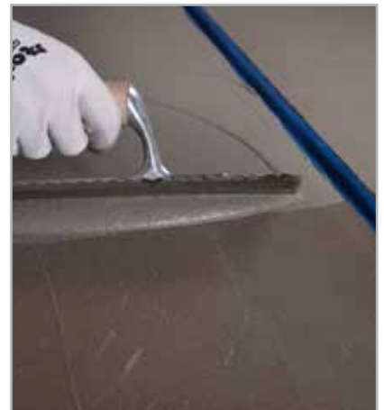
5.72 - Application of the second coat of MAPELASTIC, being careful not to let it run into the control joint
