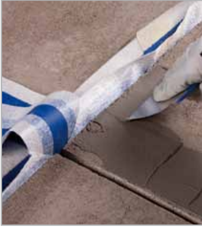
Fig. 5.67 - Insertion of upside-down “Ω” shaped MAPEBAND CROSS in the control joint and application of MAPELASTIC or MAPELASTIC SMART around the joint
