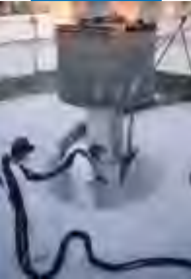
Particulars of a Purtop 1000 waterproof coating applied on various substrates (cementitious and metallic)
