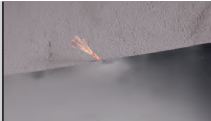
Photo 7 Electric cable previously connected to the reinforcement rods
