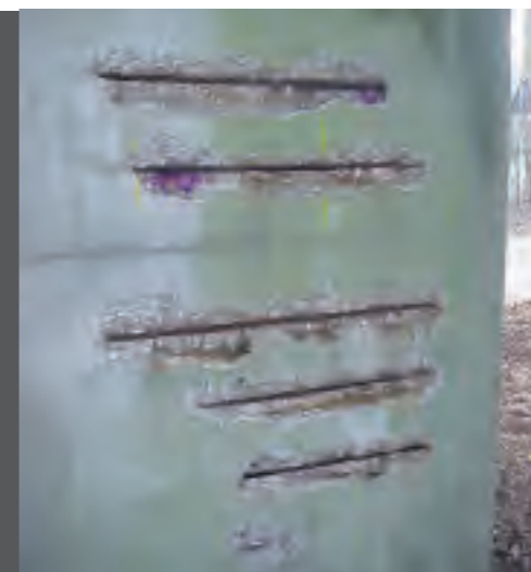
Photo 1 Deterioration of a reinforced concrete structure. Concrete detached following corrosion of the reinforcement steel due to carbonatation
