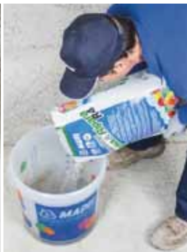
Adding Planitop Smooth & Repair to the mixing water admixed with Mapetard ES
