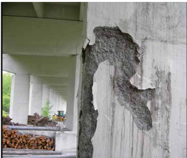
Photo 1 Example of concrete deteriorated by sulphur aggression
