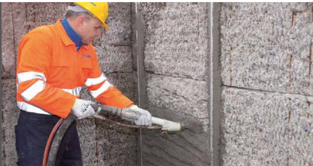
Photo 6 Application by spray of MAPEGROUT 430 , class R3 structural mortar on a concrete structure
