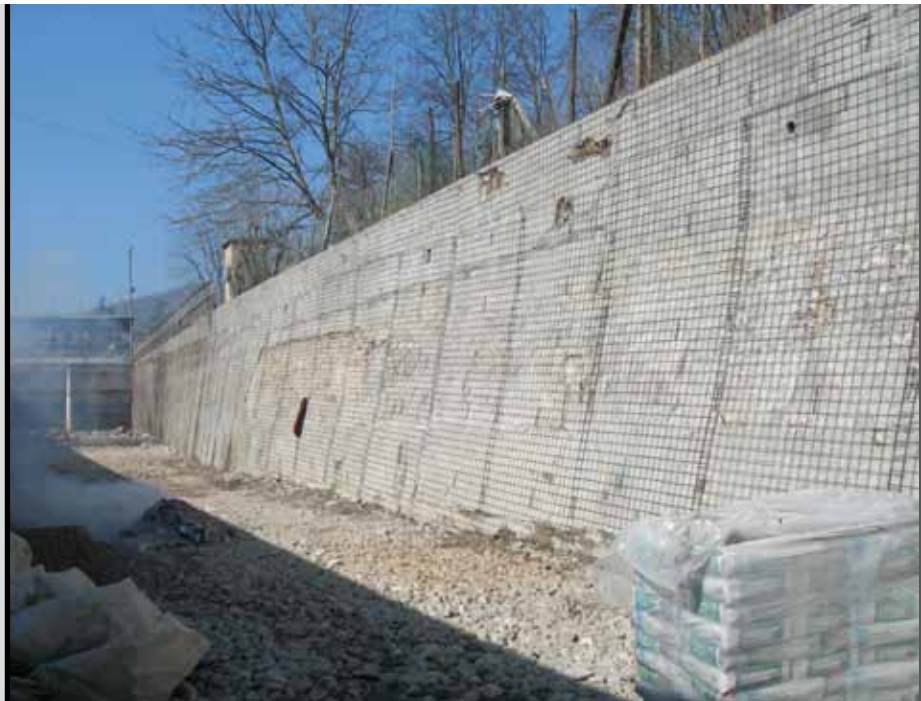
photo 2 An example of new reinforcement applied on the surfaces to be repaired
