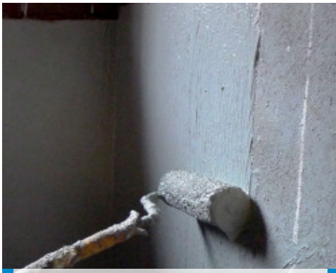
Application of Mapelastic Foundation by roller on a substrate evened out using Planitop HDM Maxi
