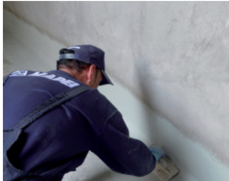
Mapelastic Foundation spread on by trowel to waterproof against water in negative pressure
