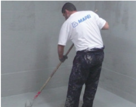
Mapelastic Foundation spread on by roller to waterproof against water in negative pressure
