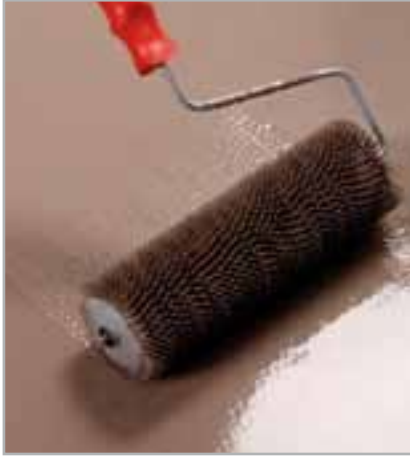
Fig. 5.4 - Application of smoothing compound and going over the surface with a spiked roller to remove any air bubbles
