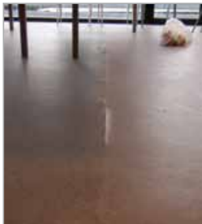
Fig. 4.7 - Unstable flooring with joints pushing together
