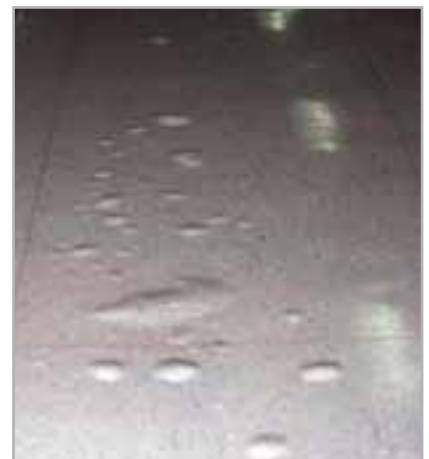
Fig. 3.3 - Formation of bubbles caused by installing flooring on a damp substrate
