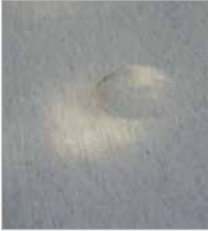
Fig. 3.1 - A substrate sinking around through pipe-work due to its insufficient thickness
