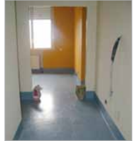
Fig. 3.12 - Installation on a substrate not levelled off sufficiently
