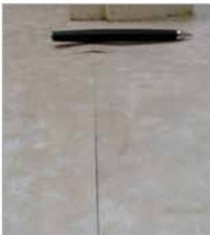
Fig. 4.8 - Unstable flooring with joints pulling apart
