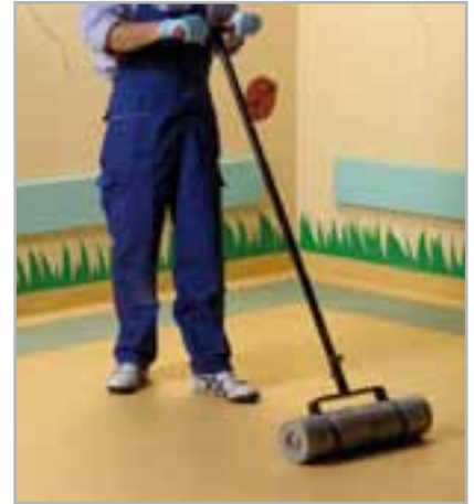
Fig. 5.7 - Going over a floor covering with a roller to remove air bubbles
