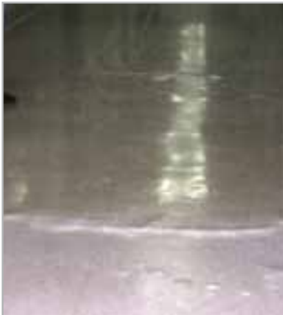
Fig. 3.11 - Swollen covering due to cracking not being sealed
