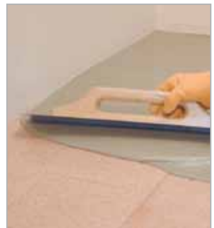
Fig. 5.3 - Application of smoothing compound and going over the surface with a spiked roller to remove any air bubbles
