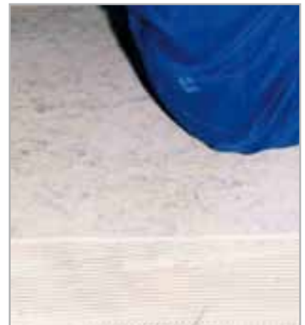
Fig. 5.8 - Going over flooring just after installation while the adhesive is still fresh
