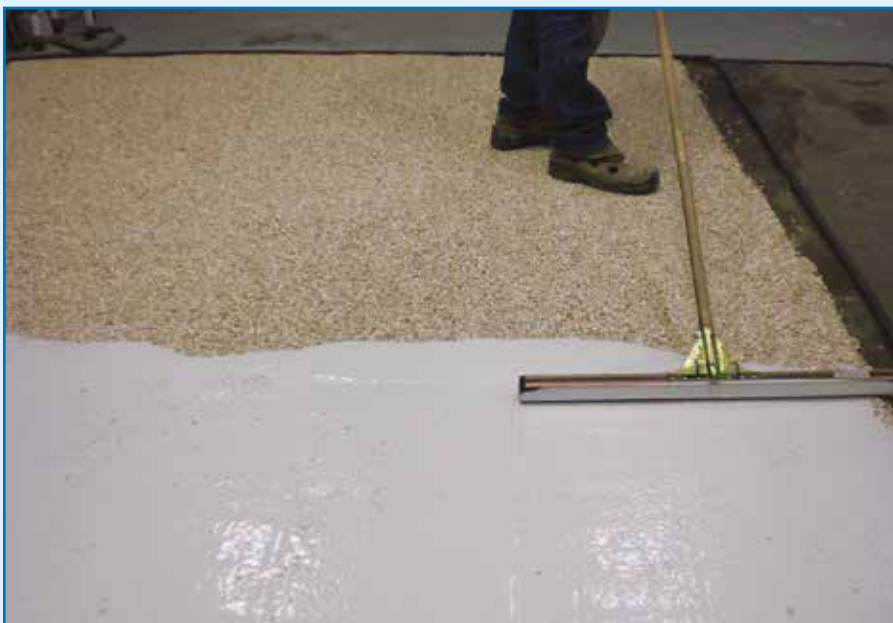
Application of Ultratop on the hardened surface of the Mapefloor 910/natural aggregates mixture
