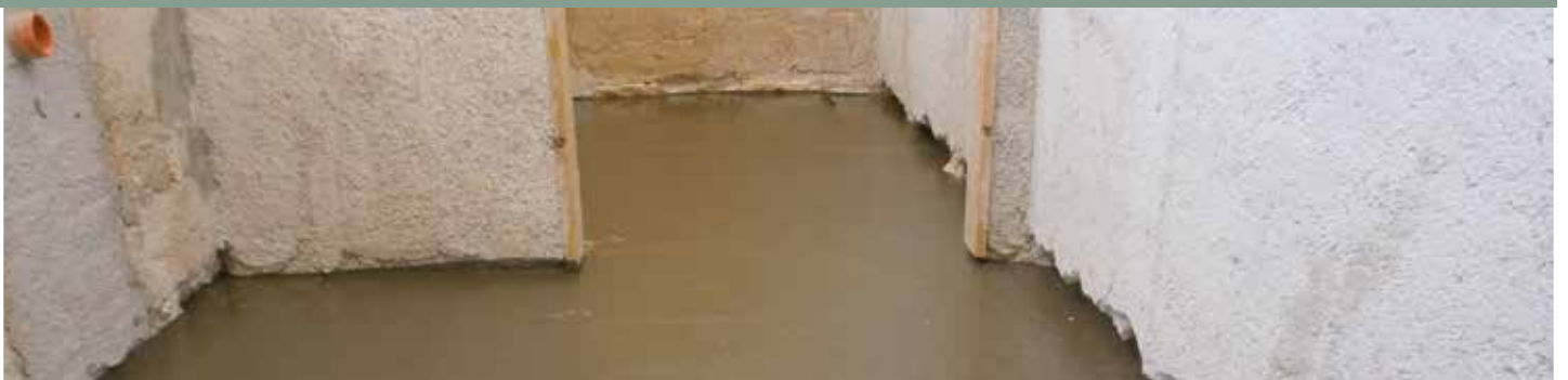
3 | Strengthening the outer face of a floor with a pour of Planitop HPC Floor Mons. Giovanni Bacile School - Bisacchino (Palermo)
