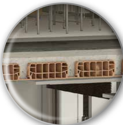
Strengthening a floor with an added layer to form a rigid plane using Planitop HPC Floor
