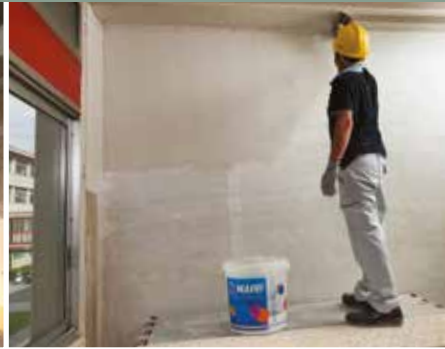
2 | Anti-seismic protection by applying MapeWrap EQ System applied on dividing walls - Teresio Olivelli Comprehensive School - Darfo Boario Terme (BS)
