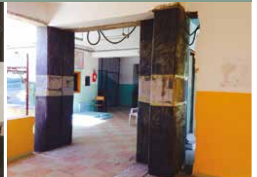
6 | Shear strengthening of pillars with MapeWrap C fabric Mirto District Elementary School - Crosia (Cosenza)
