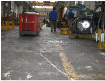
Typical example of damaged and oil-impregnated surface.
