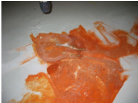
Typical color deviation due to concentrated sulphuric acid attack.
