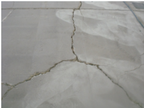
Shot blasting treatment made cracks deeper and wider and removed all loose and friable parts.
