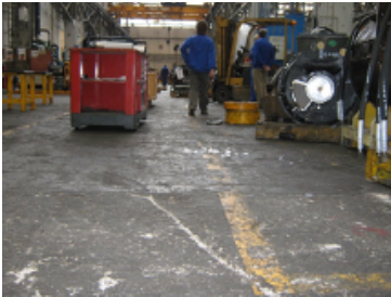
Typical example of damaged and oil-impregnated surface.
