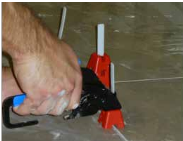
Figure 2: Example of a thin-body tile being installed using a mechanical edge-leveling system to reduce lippage
