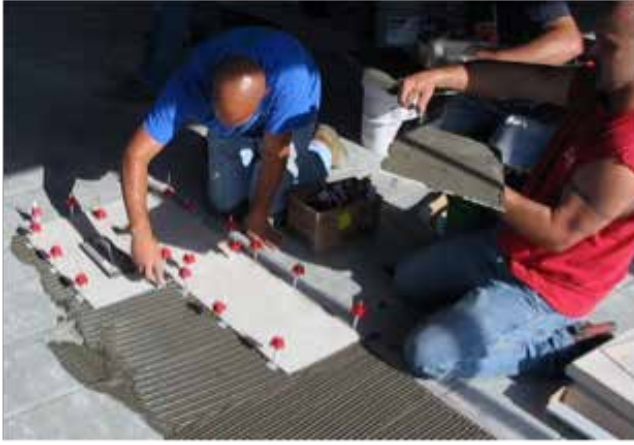
Figure 3: Example of thin-body tile over existing tile during a renovation using a mechanical edge-leveling system
