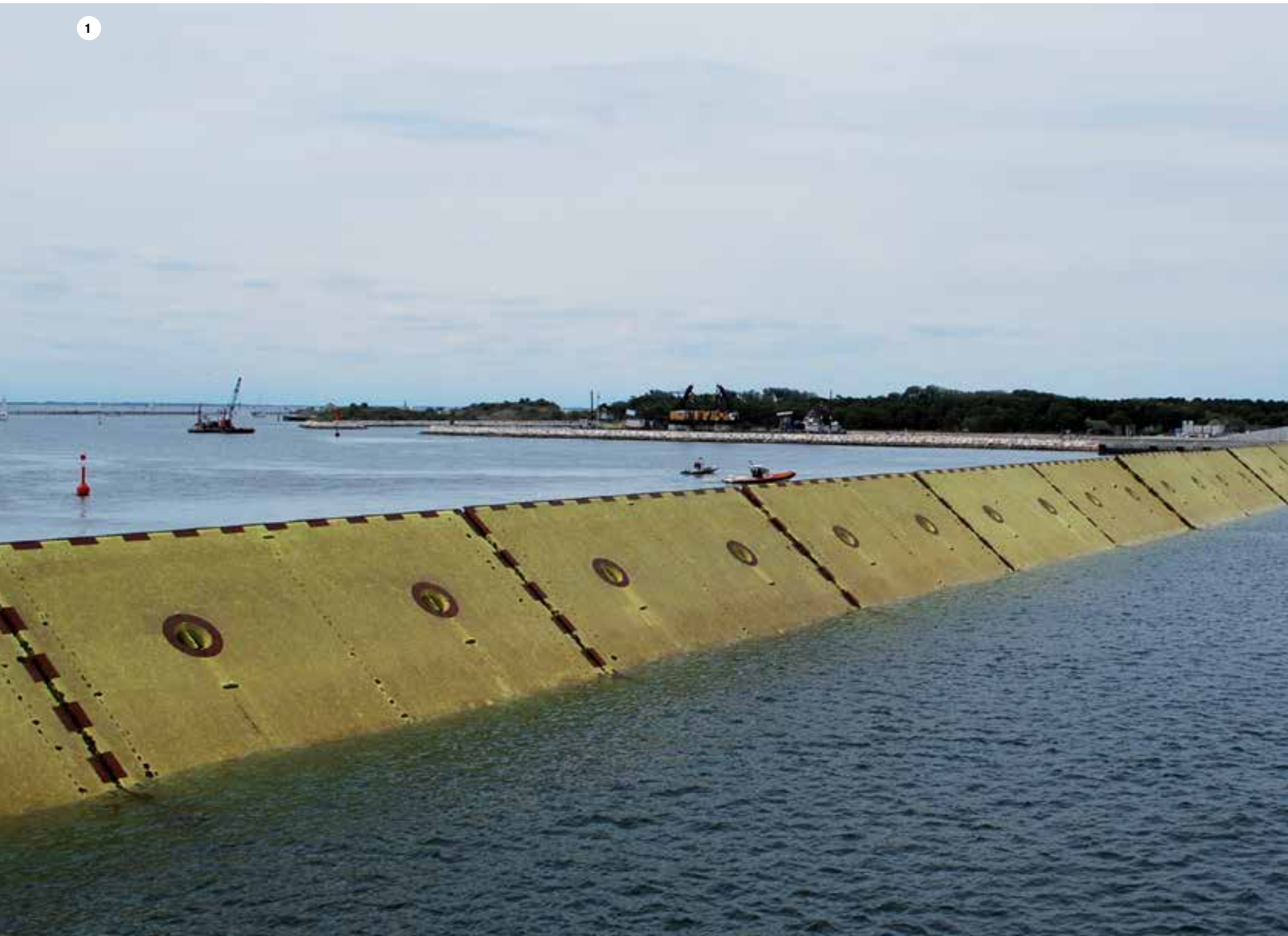
1. The floodgates being maneuvered into position at the entrance to the port of Chioggia
