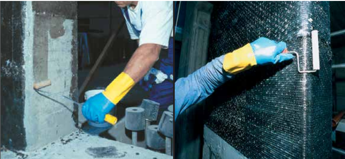
“Dry layup system”
