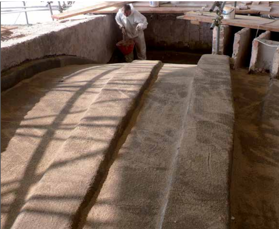
Seeding MapeWrap C Uni-Ax 300 with sand aggregate in preparation for the protective coating
