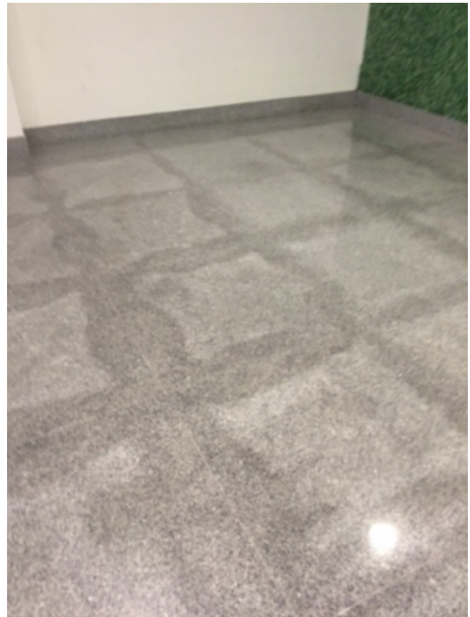
The unsightly “picture framing” effect on this granite floor could have been prevented by using epoxy setting materials or by sealing all six sides of the tiles before installation.
