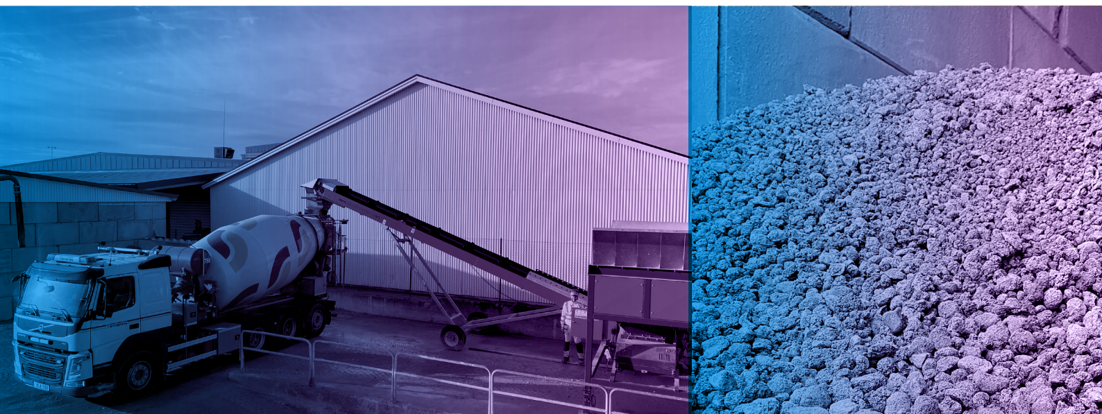
Above, left - Simple feed hopper and conveyor solution to feed dry washing aggregates into a dirty truck.
