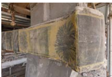
Reforço do tirante com tecnologia FRP System. Tie-rod strengthened with FRP System technology.
