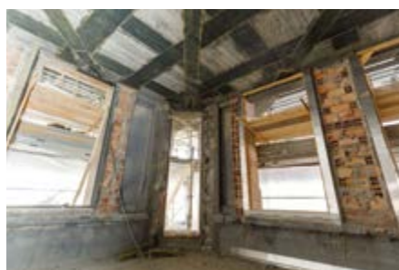
Reforço à flexão de laje com FRP System. Flexural strengthening of a floor slab with FRP System.
