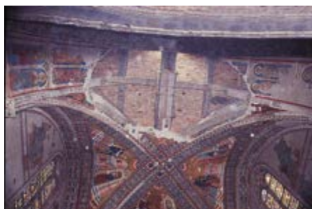
Danos na abóbada após o terremoto. Vault damage following the earthquake.
