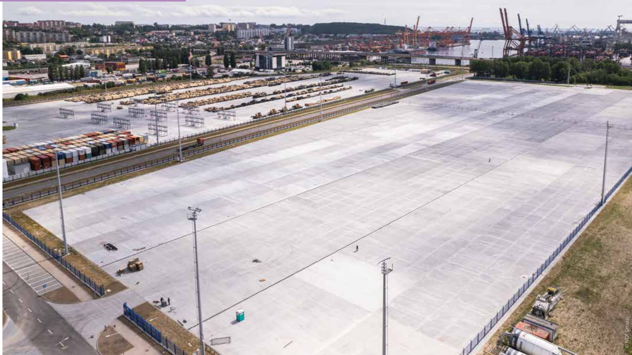
LEFT. Storage yards covering an area of 18.6 hectares were constructed in the Port of Gdynia. Concrete floors were completed with Mapei fibers and admixtures.
