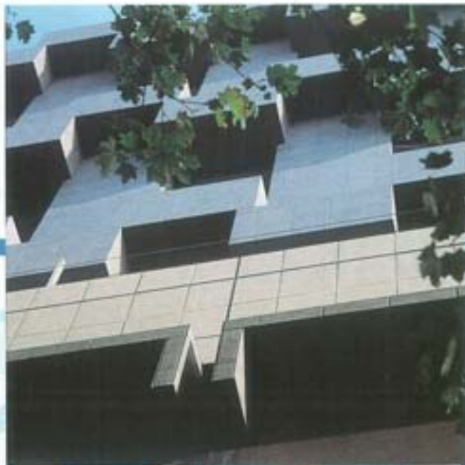
At left and on opposite page, details of the facade with its eye-catching porcelain tile cladding
